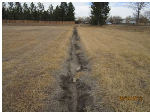
Figure 2: EDB trickle channel filled with sediment
